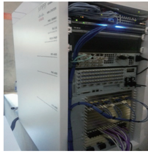
Switcher Rack System
