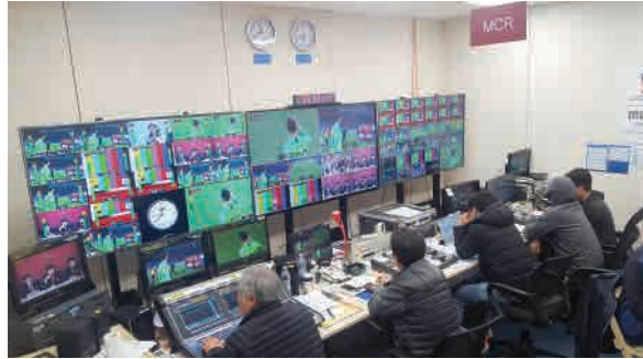
MBC MCR (Control Room)
