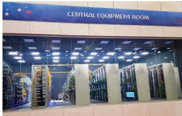
CER (Central Equipment Room)
