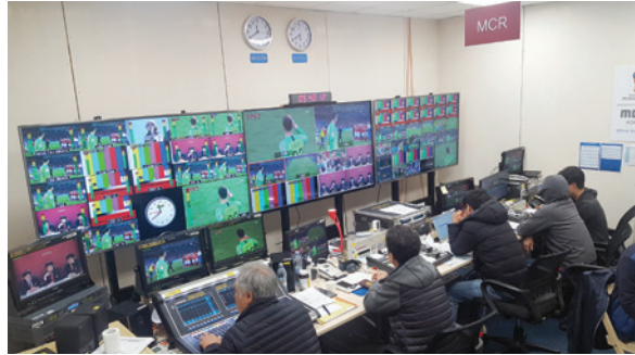
MBC MCR (Control Room)
