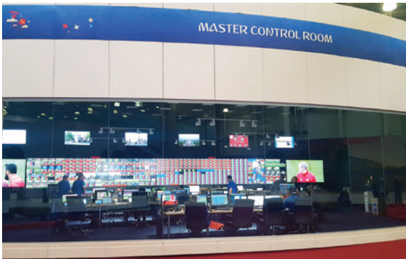
MCR (Master Control Room)
