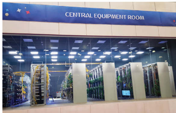
CER (Central Equipment Room)
