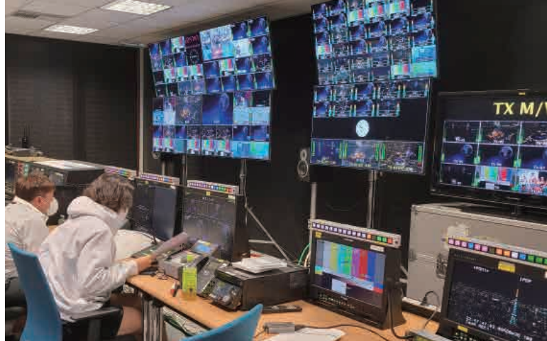
MCR(Master Control Room)
