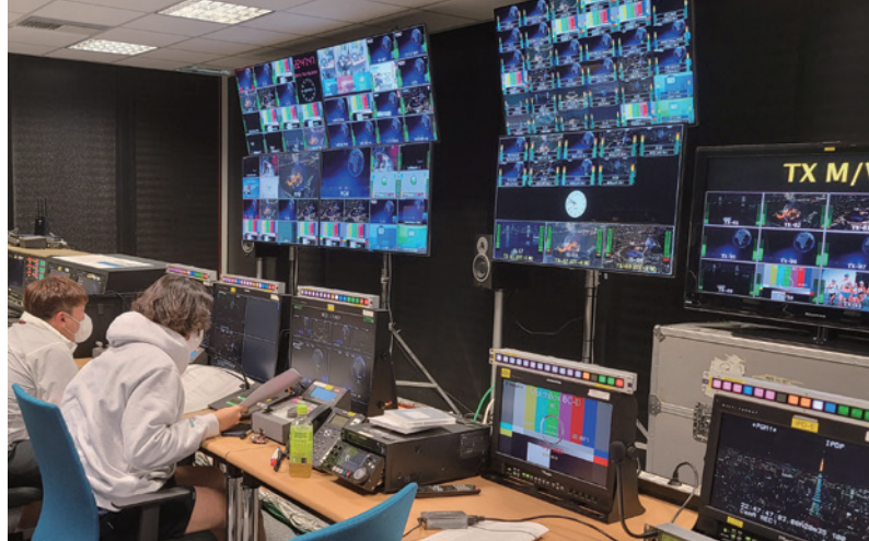
MCR(Master Control Room)
